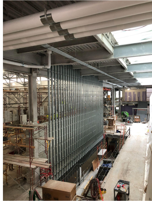
Framing of Logo Wall in Canyon. Right Photo - also see skylight almost completed
